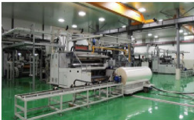
Figure 5: New CPP Production Lines in Melaka
