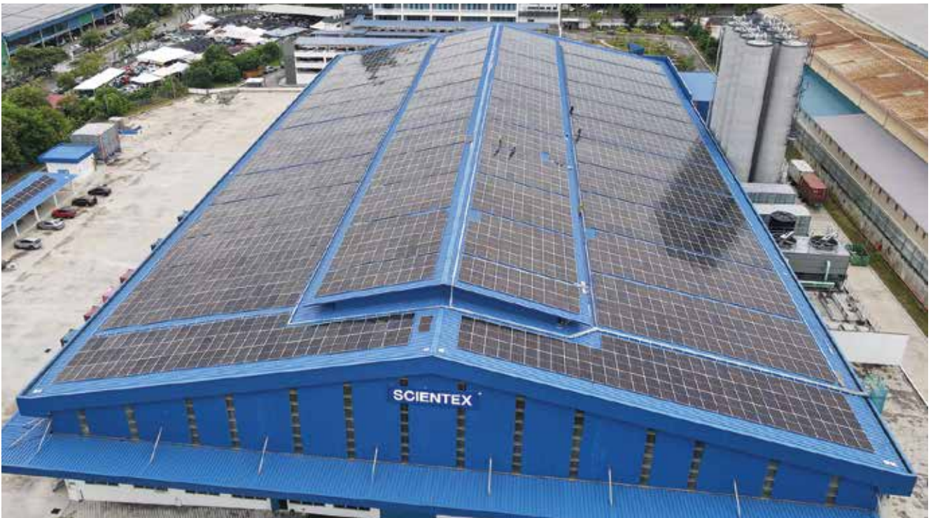
The solar PV system under construction at one of our key manufacturing plants
