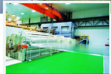
BOPP film stretching plant
